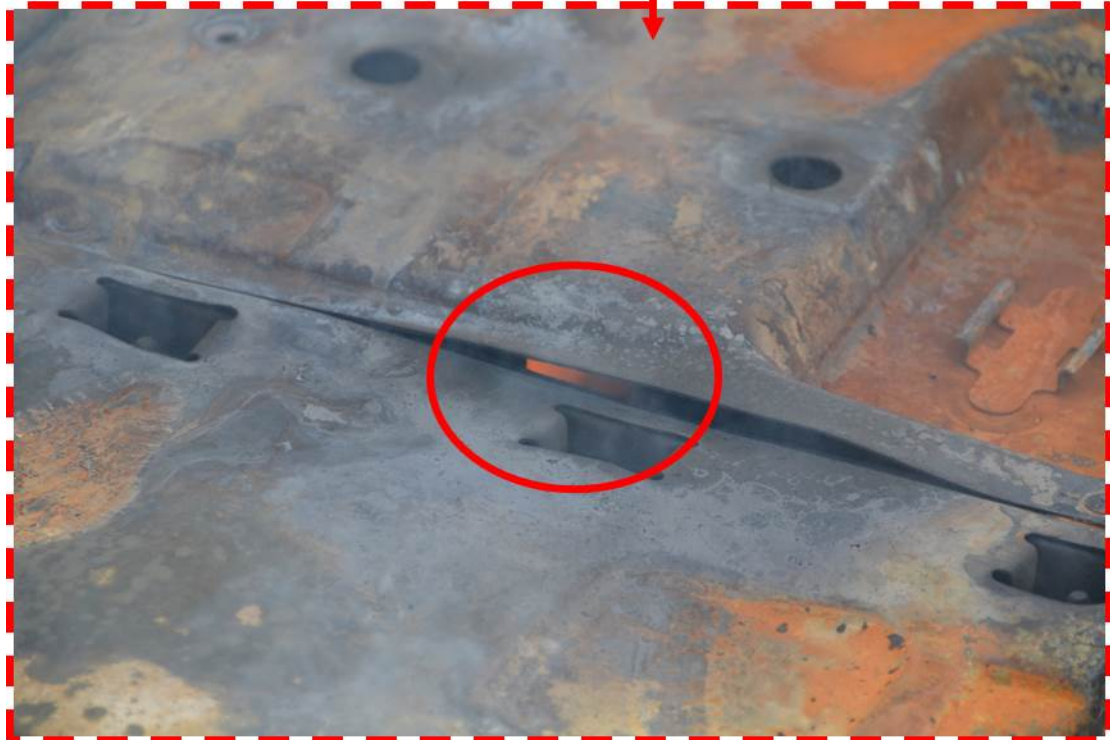
Figure 73 Reignition of Battery A3 approximately 22 hours after the conclusion of the test (flame circled red)
